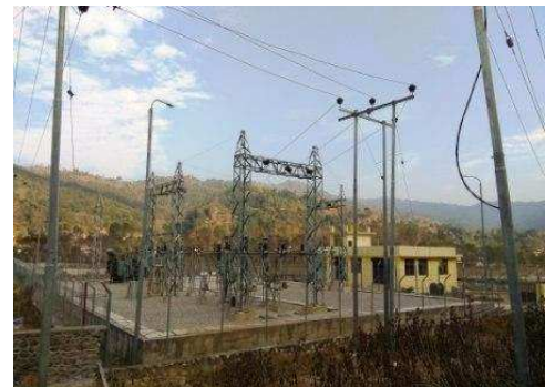
Construction Power Substation
