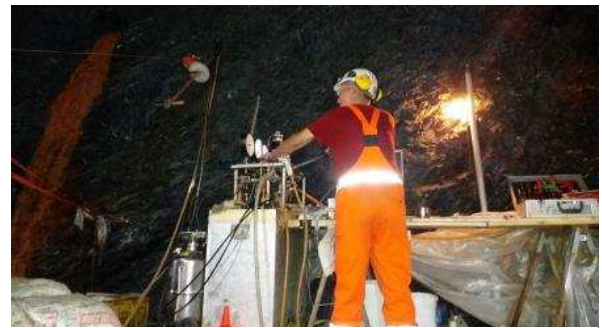
Slotter test inside Power house
